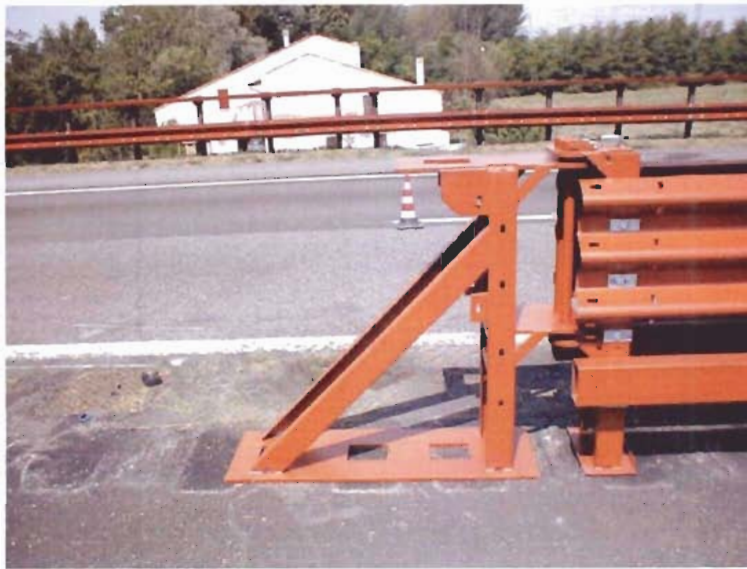
Figure 7 – Positioning of backup support
